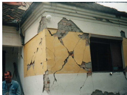
Figure 1. Damage of two store building from Kolubara region, Serbia
